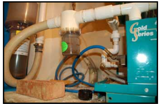
In order to qualify for the Ohio Good DEED program, an ISO 11143 compliant amalgam separator like the Solmetex pictured above must be in use in dental offices that place or remove amalgam.
