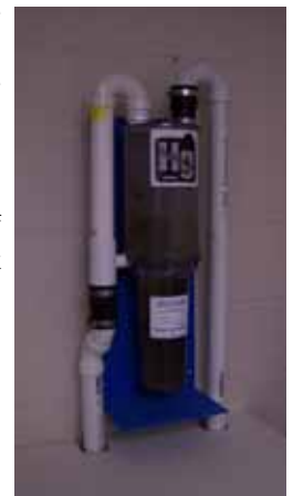
One of five Solmetex amalgam separators at CWRU which enables the school to qualify for the Ohio Good DEED Program.
